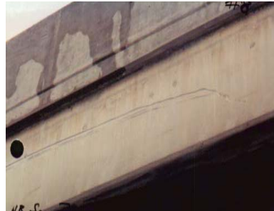
(b) typical impact damage pattern (PennDOT).
