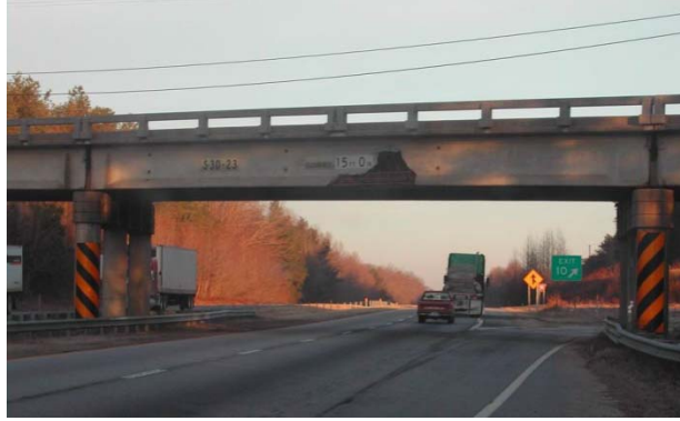
Figure 3-1 Loss of section of AASHTO girder due to vehicle impact (Harries; not taken in PA).
