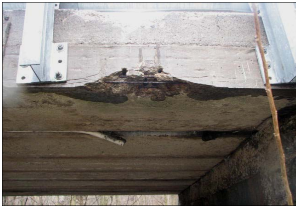
(a) spalling at original attachment and possible future damage at sight of new attachment.
