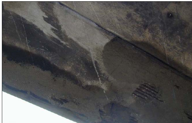
Figure 3-2 Scraping due to minor vehicle impact (Lake View Drive Bridge prior to collapse; PennDOT and Harries 2006).
