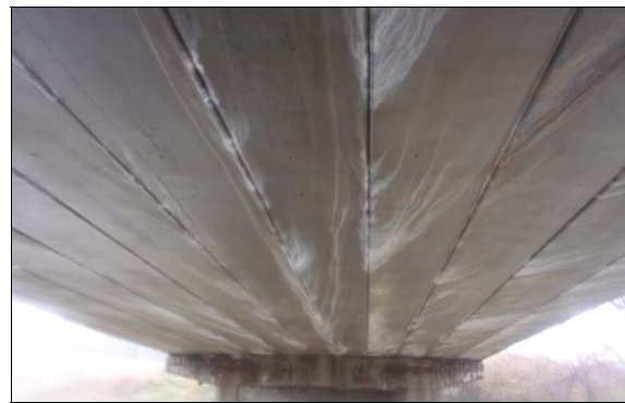
(b) water leaking between adjacent box girders (PennDOT).
