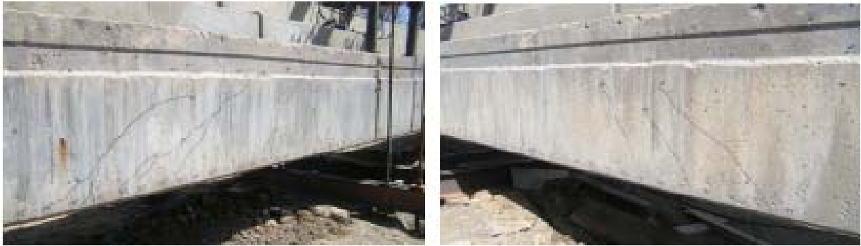
Figure 3-12 Representative shear distress (Lake View Drive EXTERIOR test girder; Harries 2006).
