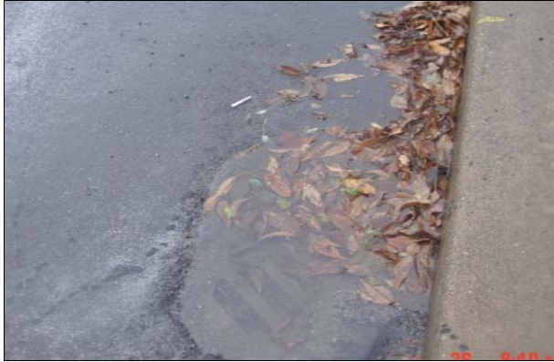
(a) water pooling due to clogged deck drain (PennDOT).
