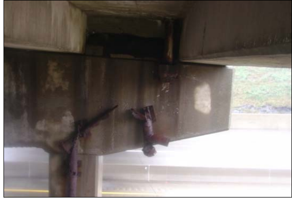
(b) damaged drain system resulting in water affecting superstructure (PennDOT).
