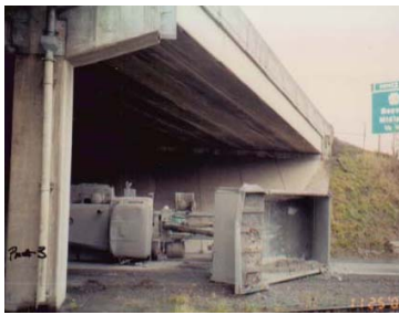
(a) following vehicle impact (PennDOT).
