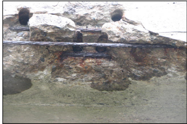
(b) unpatched holes at sight of original attachment result in exposed strands.
