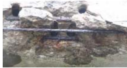
(b) exposed strands without corrosion (Fig. 3-8b).
