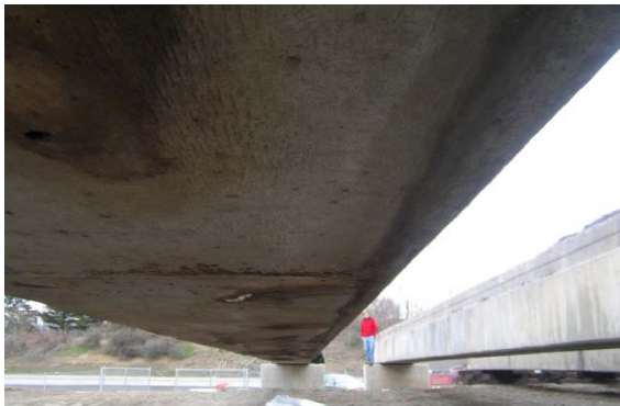
(a) water coming down exterior face of adjacent box girder (Harries 2006).
