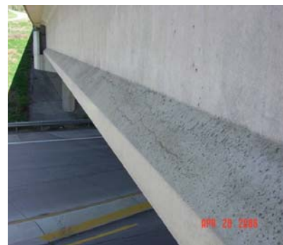
(c) longitudinal cracking resulting from impact.
