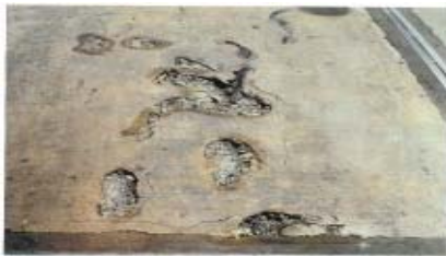
(a) concrete spalling.
