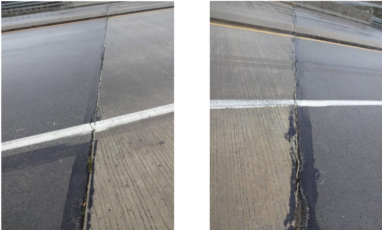
Figure C68: Cracking and erosion of edges in contact with sealant
