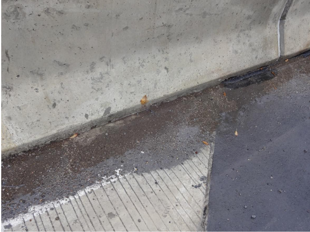
Figure C105: Minor debris accumulation along the edge of the deck
