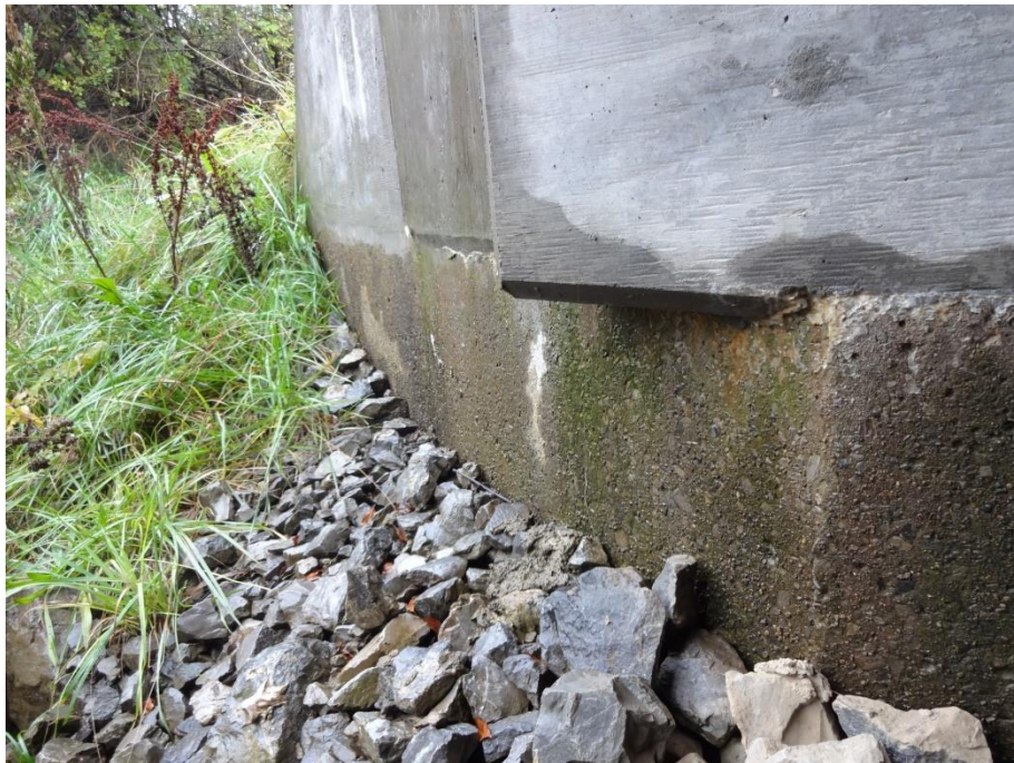
Figure C113: Severe leakage from interface of new and old abutment sections
