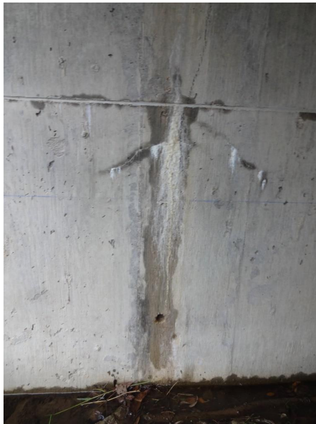
Figure C93: Leakage in cracks propagating from the abutment stem and header interface
