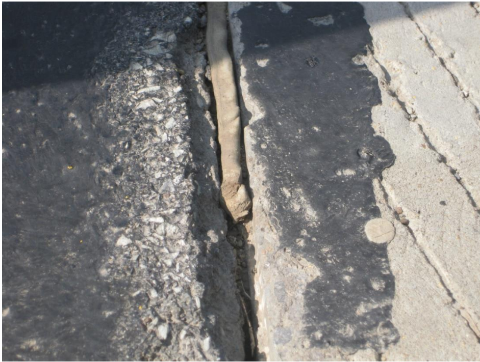
Figure C70: Close-up of damaged seal in figure C68
