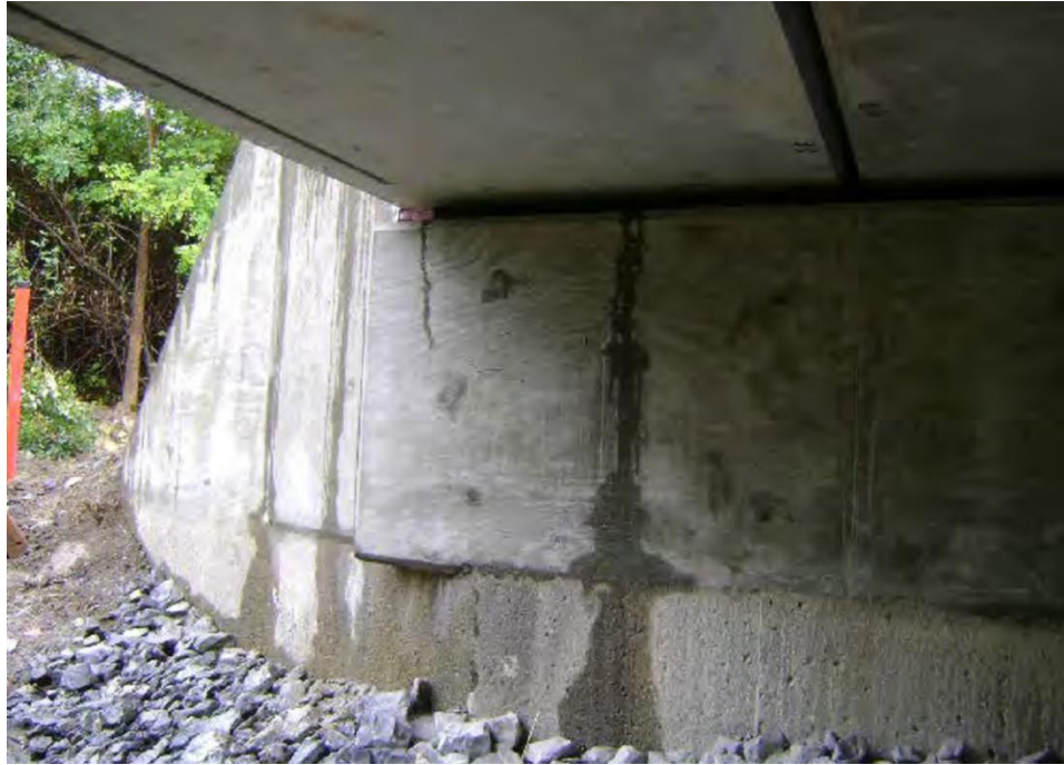
Figure C112: Staining of abutment wall observed by PennDOT inspectors
