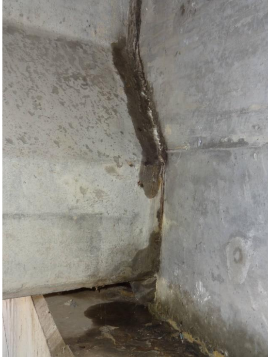
Figure C73: Leakage at interface of abutment backwall and beam
