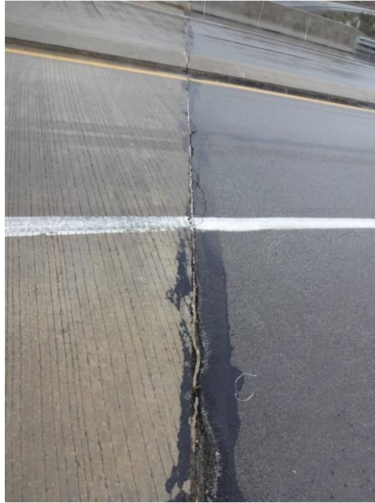
Figure 4.4: Cracking and erosion of joint edges
