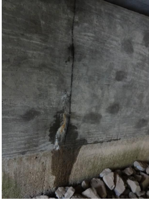
Figure C114: Leakage at cracks originating from interface of new and old abutment sections
