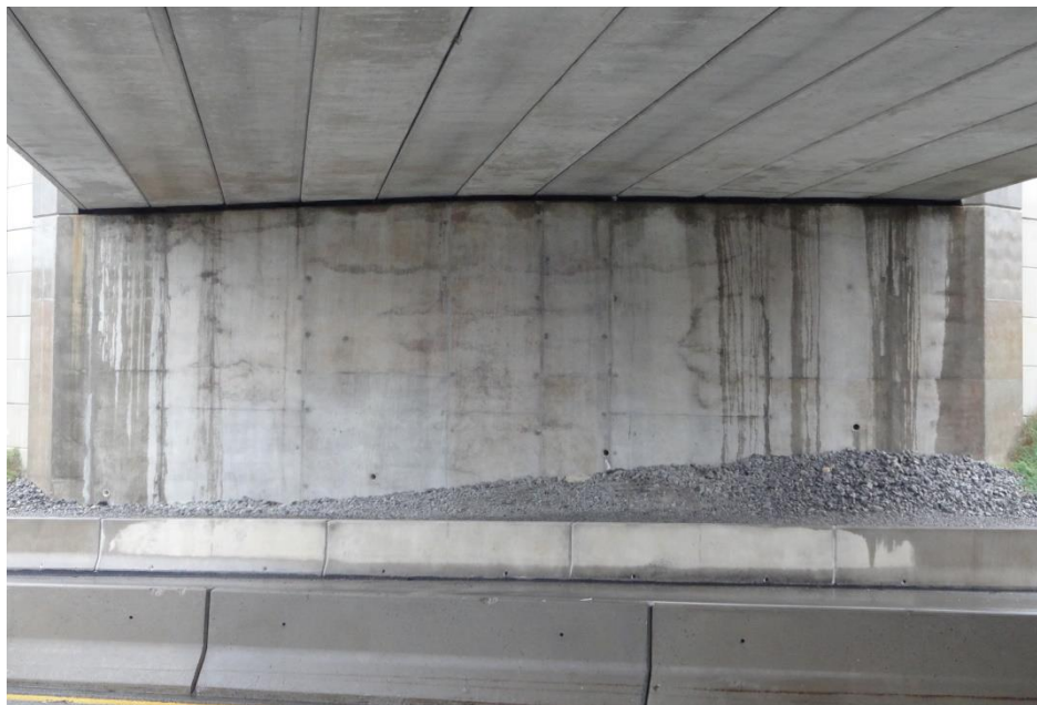
Figure C83: Water staining on abutment
