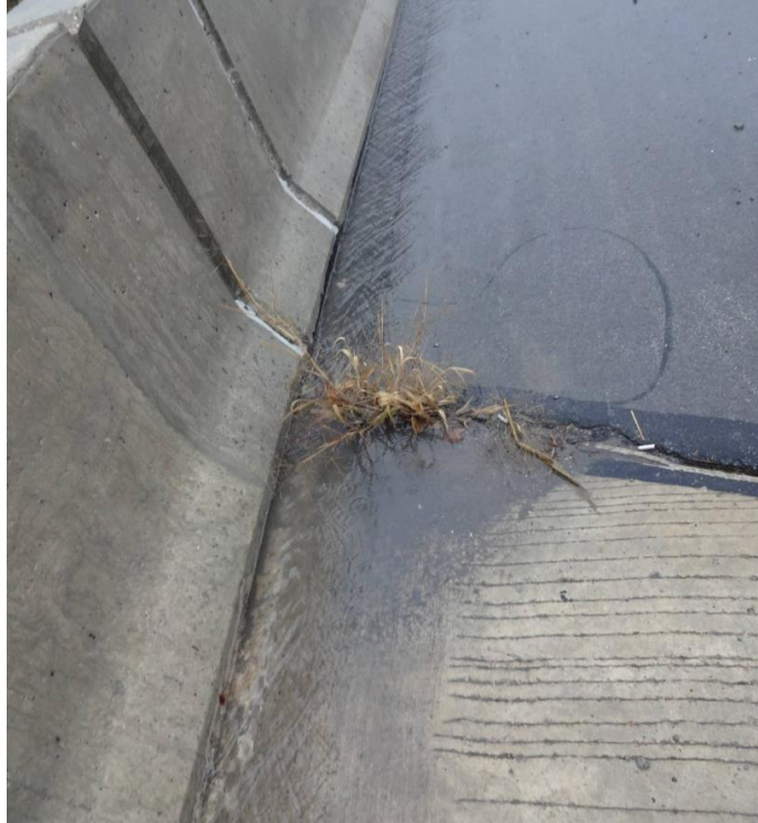
Figure C75: Detour of part of discharge into joint
