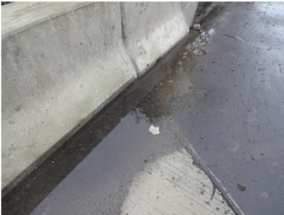
Figure C95: Silt deposition with lack of flow of water along deck edge
