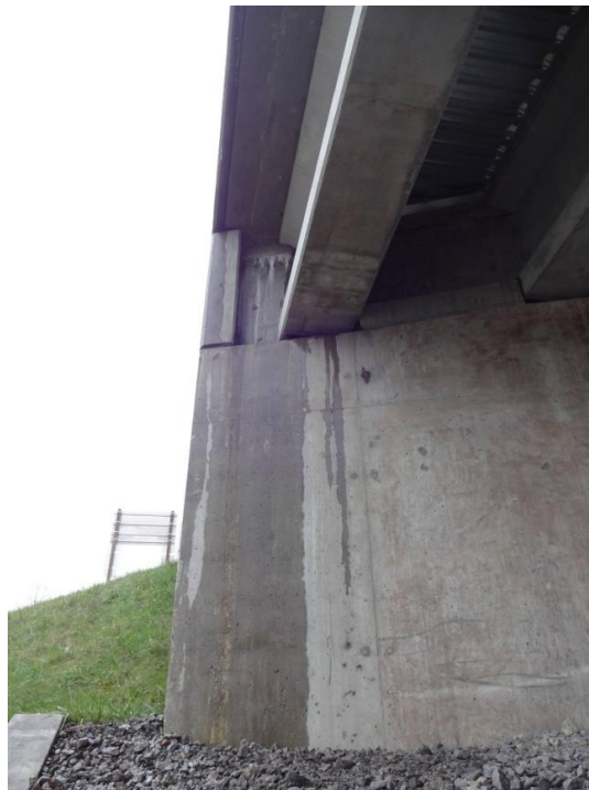
Figure C74: Leakage at edge of abutment
