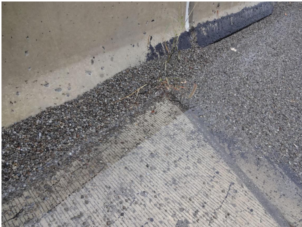
Figure C86: Water ponding at the edge of the deck near the expansion joint
