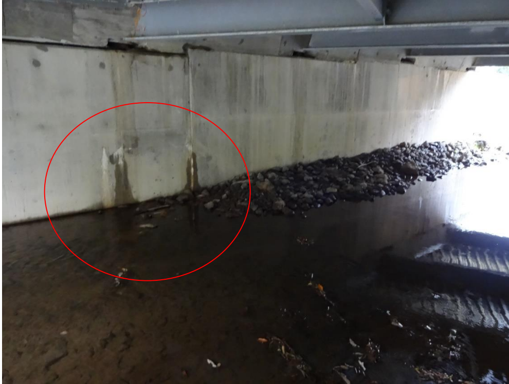
Figure C94: Leakage through cracks with efflorescence
