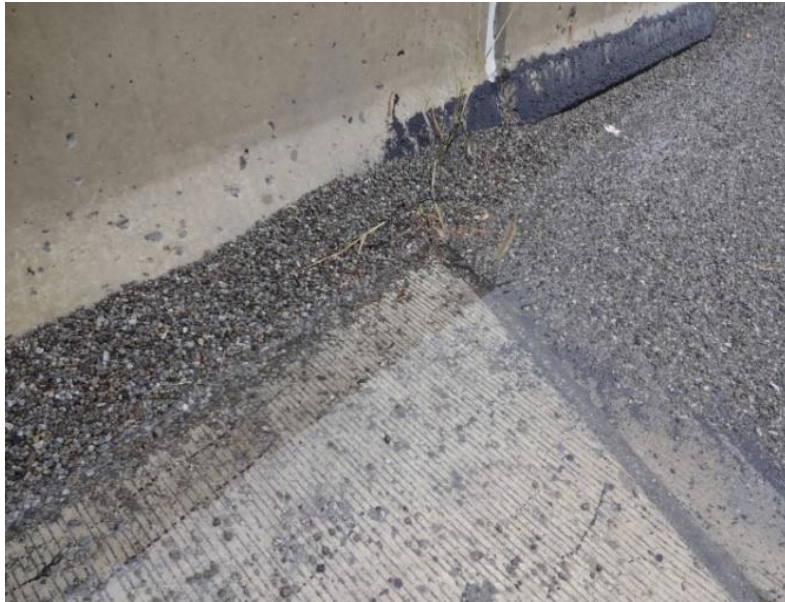
Figure 4.16: Debris accumulation causing water ponding – Prospect #1 Bridge
