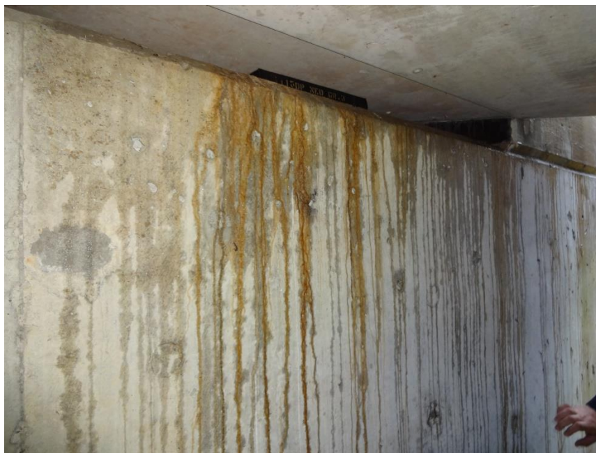
Figure C102: Severe water staining on abutment wall
