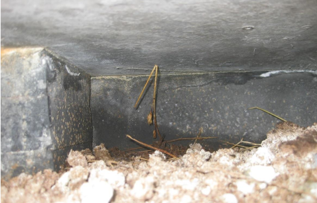
Figure C85: Water staining on top and bottom of back wall on abutment seat
