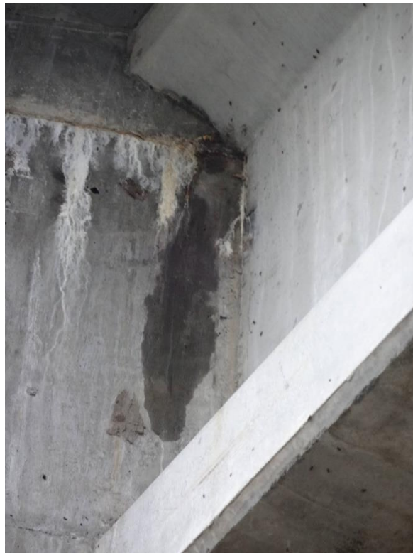
Figure C72: Leakage at interface of abutment backwall and beam
