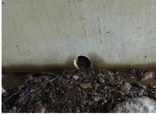
Figure C96: Silt deposition in weep hole
