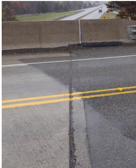
Figure C82: Maintenance works overlapping on expansion joint and deterioration of concrete edges
