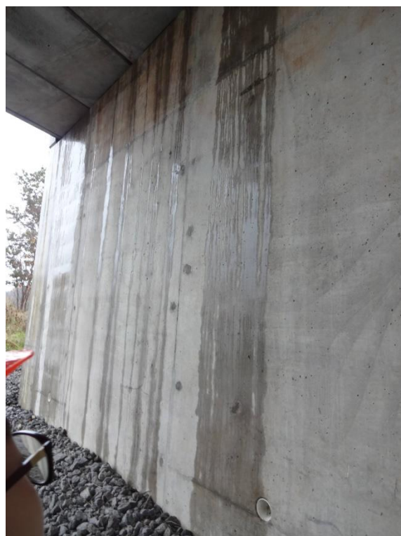
Figure C84: Severe water staining on edge of abutment wall
