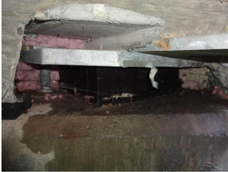
Figure C92: Leakage in bridge abutment seat
