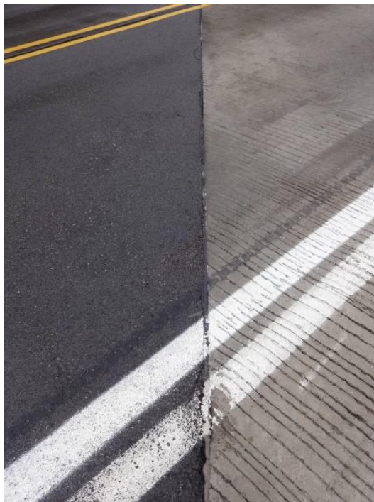
Figure C101: Slight deterioration of HMA surface adjacent to joint
