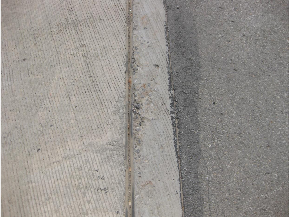
Figure C80: Moderate debris accumulation in expansion joint
