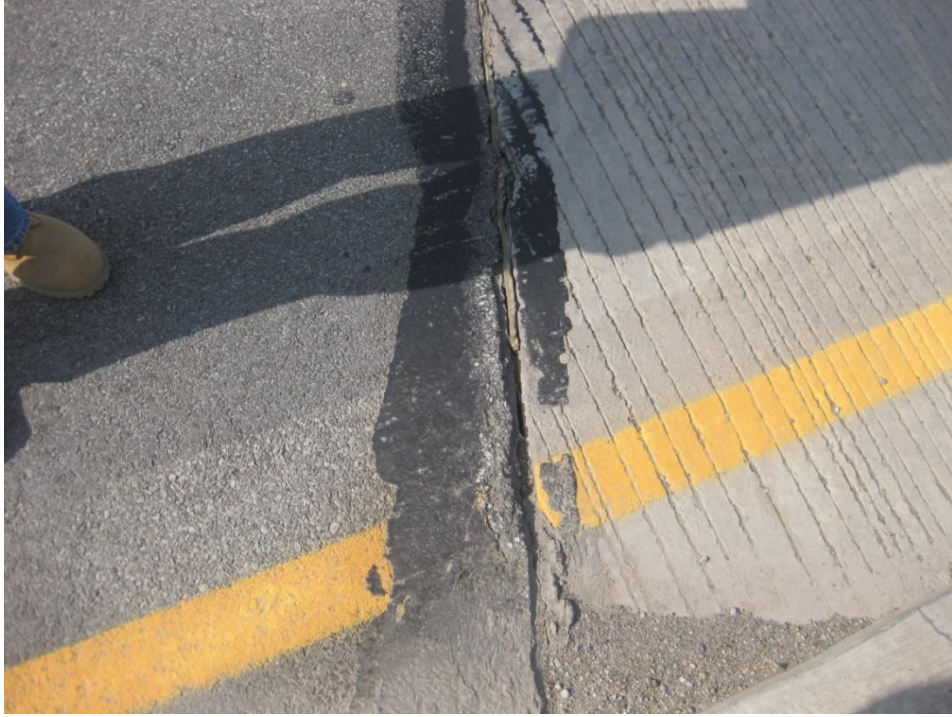
Figure C69: Damaged Silicone sealant seal
