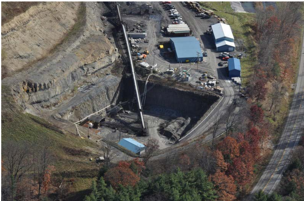
Figure 2.3: Box-cut development at the portal entries of Little Toby in Elk County, PA (Rosebud Mining 2006).
