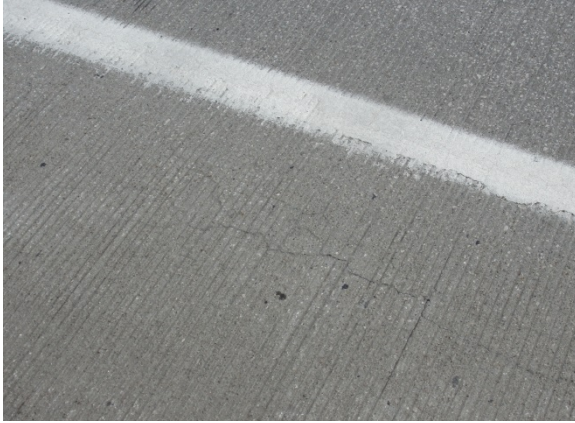
a) Minor hairline cracks (Bridge A)
