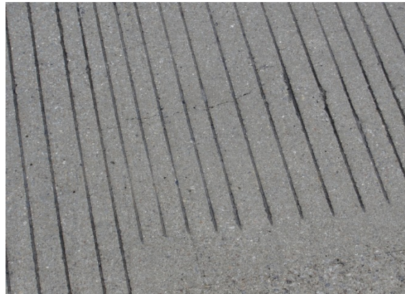
d) Minor Hairline Cracks (Bridge D)
