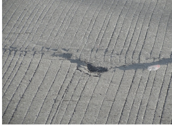
b) Apparent Pop-out of LMC (Bridge F)
