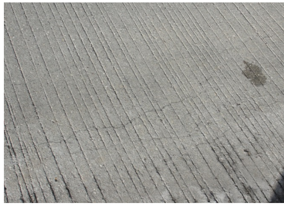
f) Hairline Longitudinal Cracks (Bridge F)
