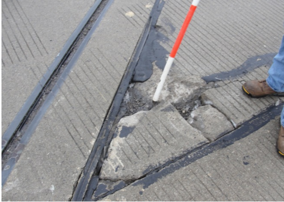
a) Damage to LMC overlay at location of acute skew (Bridge D)
