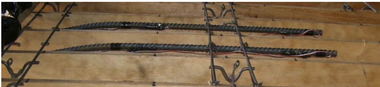
(f) Photo of cranked bars (S-18-B and S-6-B shown) prior to casting concrete.
