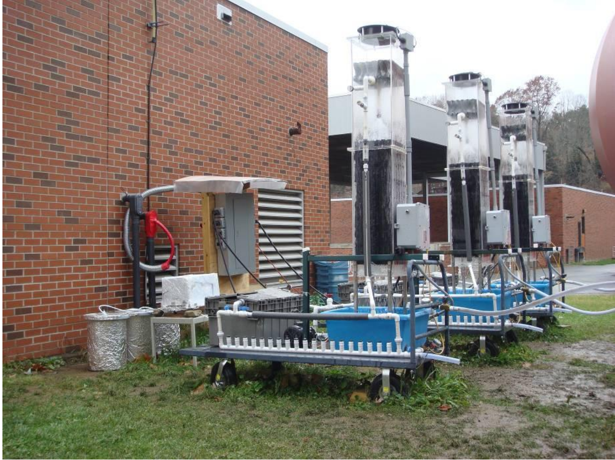
Figure 2.3. Pilot-scale cooling towers, which were modified to withstand the outdoor environment.
