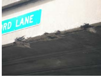
b) Impact damage to fascia beam of Crawford Lane over I-70. [Kasan]
