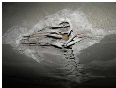
(b) Soffit and fascia of McIlvaine Road bridge over I-70 damaged by vehicle October 18, 2010 (PennDOT)
