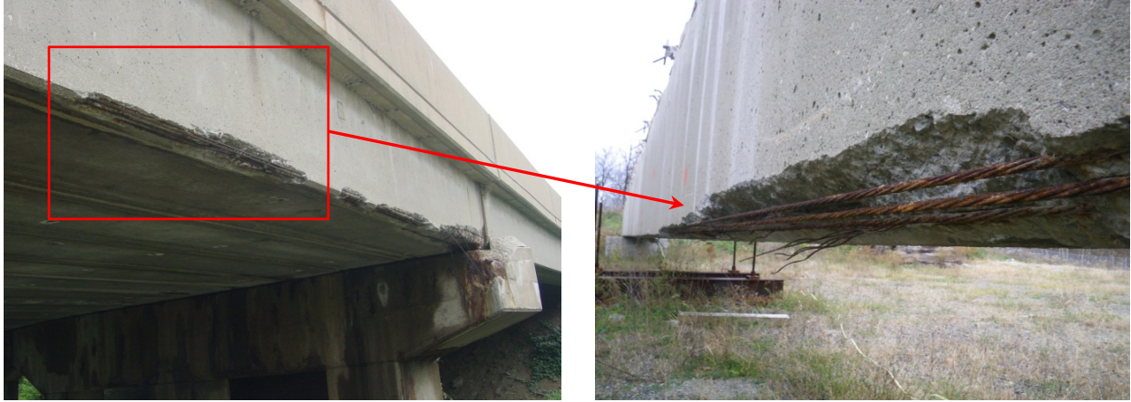
a) prototype girder in situ (photo from PennDOT inspection report dated August 8, 2007).
