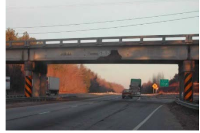
c) Bridge over I-26 north of Columbia SC showing evidence of significant vehicle impact. [Harries]
