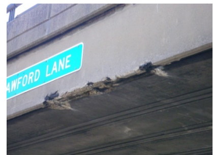
(c) Crawford Lane bridge over I-70 damaged by vehicle impact March 15, 2011 (photo by author).
