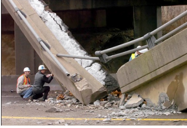
a) Lake View Drive collapse onto I-70. Impact damage led to significant strand loss, subsequent corrosion and eventual collapse under girder self-weight. [Pittsburgh Post-Gazette]
